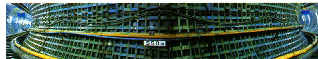
This photograph shows a 6.14 mφ tunnel with a curve radius of 20 meters which was constructed with an articulated shield machine.
