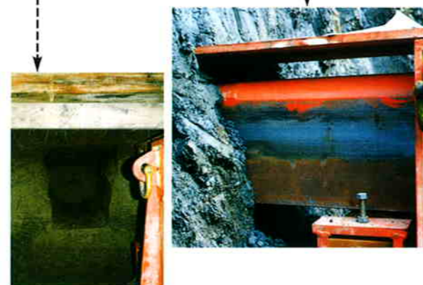
Cutter movable hood penetration
